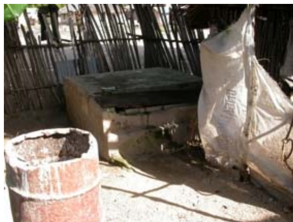
Covered well without apron
