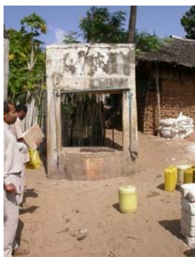
Figure 6 Protected well no apron,
