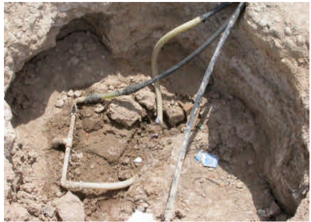
Figure 14 d: Illegal tapping on a secondary line
