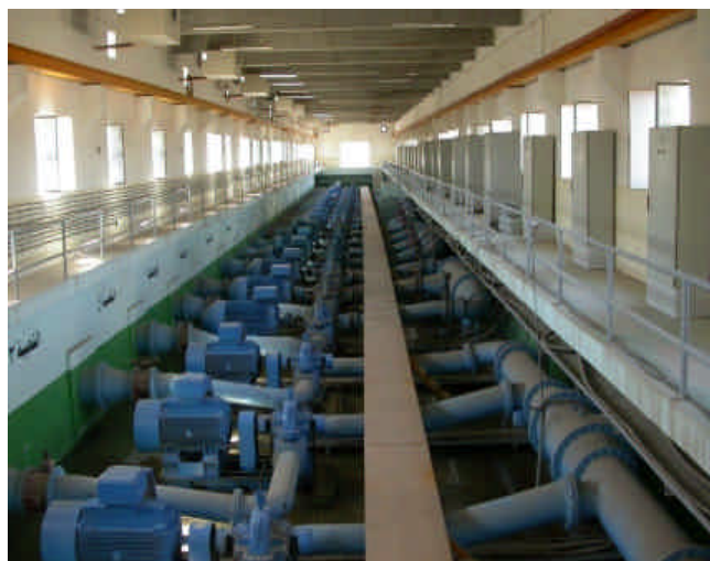
Figure 4: High lift pumps room at Wafa el Qaeda (R-zero)
