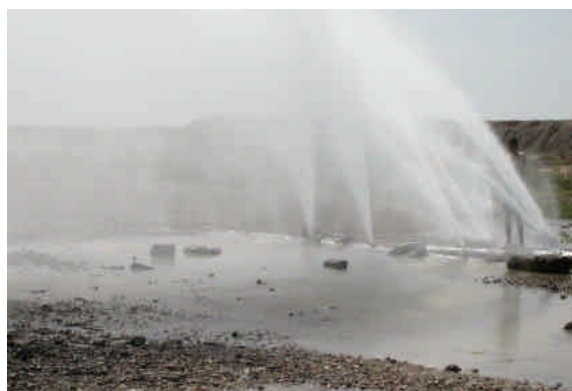
Figure 13: Leaks at the treated water pipeline to Al Shuaiba
