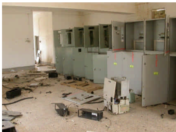
Figure 9: Damage by looters at the circuit breakers transformers control boards at PS2
