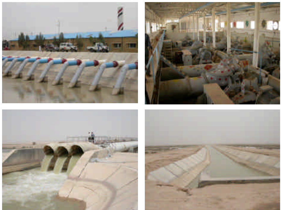
Figure 3 a,b,c,d: Intake at PS2, diesel and electrical pumps, pipeline over the Saddam river and open channel to R-zero. The low output is easy to observe (20-04) close to 1.5\text{m}^3/\text{s} and the consequent low level of the water in the channel is also visible
