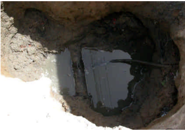
Figure 14 e: Poor collar connection
