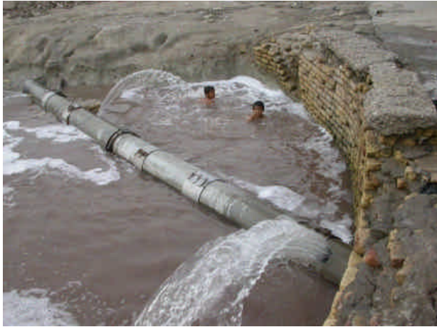
Figure 15: Leaks in the asbestos-cement pipe behind the General Hospital
