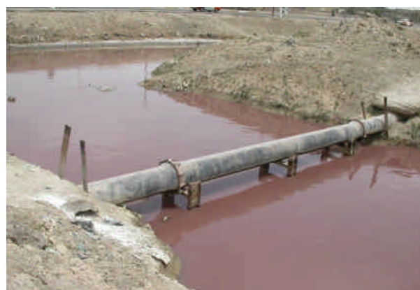
Figure 8 a, b: Canal crossing where damage may be easy, but also easy to spot
