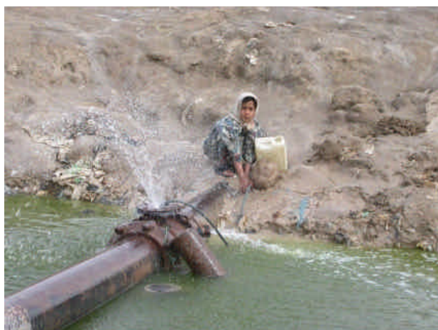
Figure 14 a: Air valve leak on a primary network pipe
