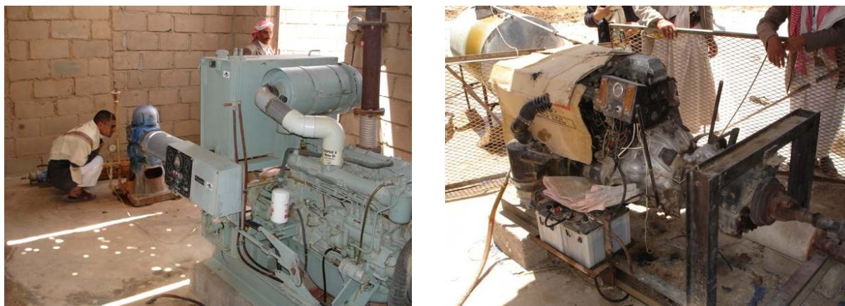
Figure 5 Pumping assembly at the al Rodwan station and at the Al Zeelah borehole.
