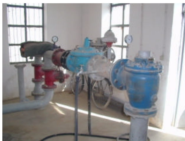
Figure 15b Afshar well field. Pumping Station.
