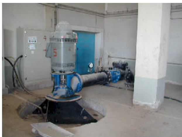
Figure 24 High Lift pump (400 kV/ 185 kW)
