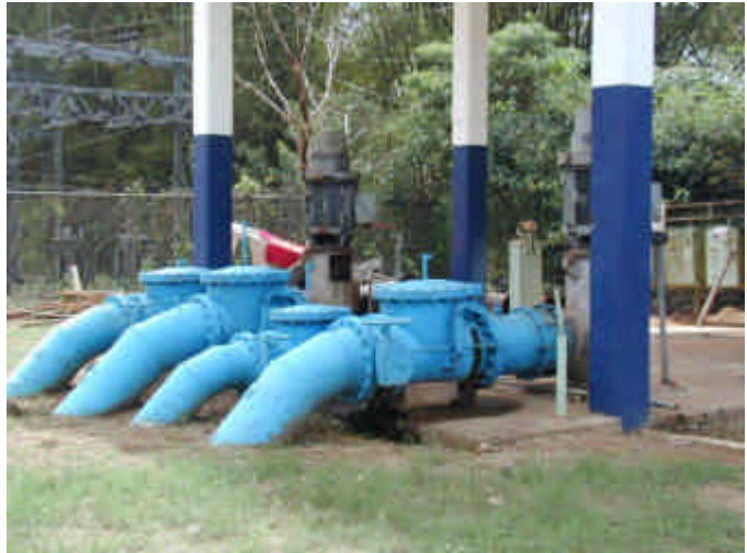
Low lift pumps
