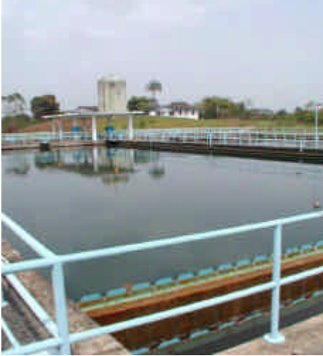
Backwash tower and sedimentation basin
