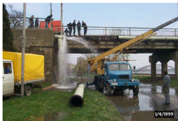
Figure 24 a,b Repairs are carried out after the destruction of the steel bridge (Varadinsky) to stop losses. The 450mm pipeline is out of repair and lies with the steel structure in the Danube
