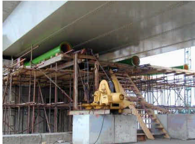
Figure 32 Conveying pipelines under the new Varadinsky Bridge
