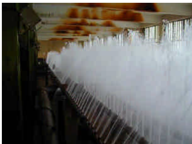
Figure 5 Aeration room to remove iron at the WTS
