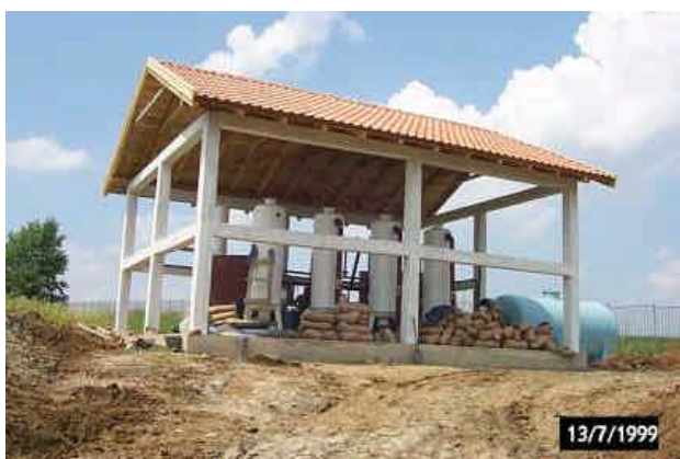
Figure 12 Treatment unit to remove iron concentration
