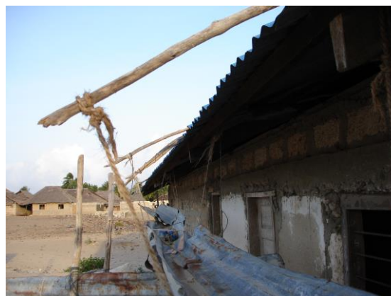
Faza poor conveying step
