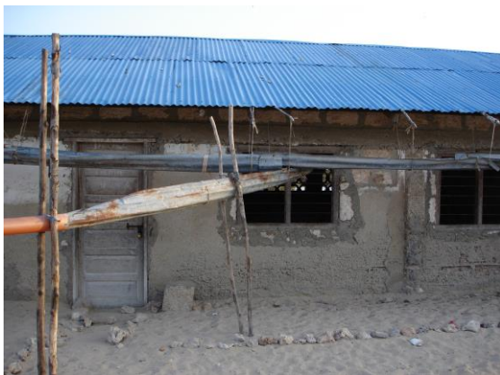
Faza School poor conveying system
