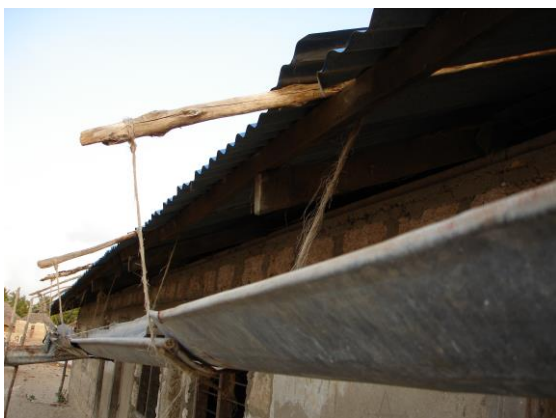
Faza School poor conveying step
